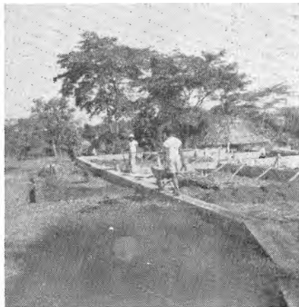
Foundation being laid for duplex at Bomi Hill which will house some of our Missionaries.
